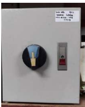
4P 80A Isolator Socomec with board
