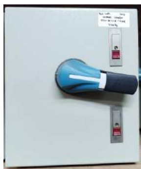
4P 250A Isolator Socomec with board
