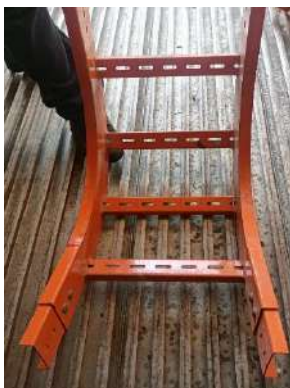
INTERNAL CABLE LADDER
